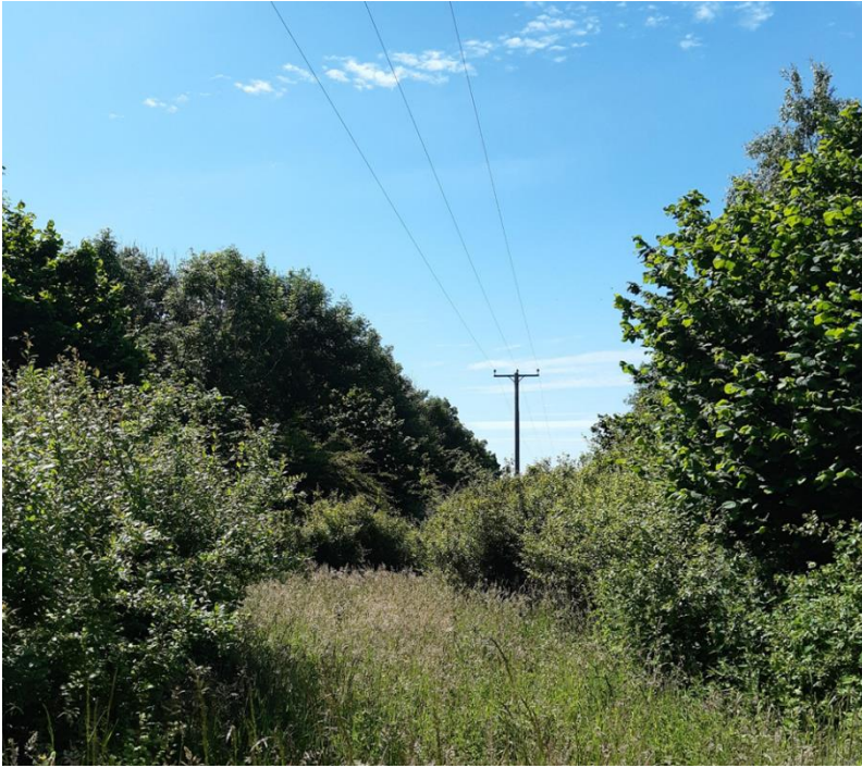
A view of HV power lines with W1 and W2 to either side.
